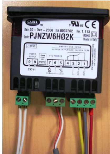
Thermostat CAREL (W6020.1) câblage existant
